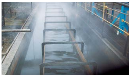
Flooded: tracker rollers in operation under water
