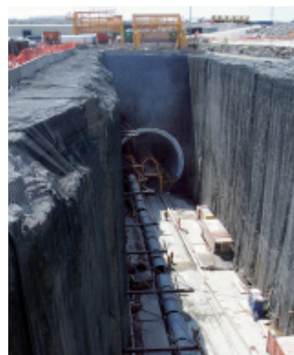
The tunnel under the City of Niagara Falls has been drilled since the year 2005 – its completion is scheduled for this year
