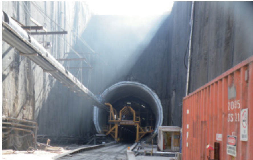
The entrance to the monster tunnel, which will be over 10 km long
