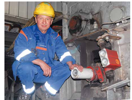
Bjarne Sørensen at one of the numerous belt conveyor systems at the combined heat and power plant in North Jutland, Denmark.
