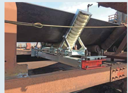
One of the HOSCH tracker rollers in action on the new belt conveyor at the steel works in Port Talbot.
